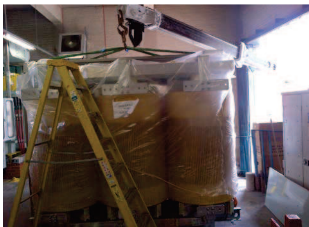
Inverter transformer delivered to Cloudesley Road Substation
