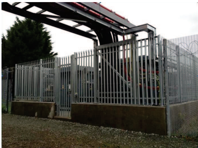
Two 2.5MW Transformer Rectifiers at Hornchurch
